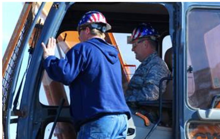
Col. Brad Webb, 1st Special Operations Wing commander, knocks the first blow to the building that formerly housed the 20th Special Operations Squadron and wing plans and programs in a demolition Dec. 6. A new crash/rescue facility for the 1st Special Operations Civil Engineer Squadron Fire Emergency Services Flight will be built at the site. (U.S. Air Force photo/Airman 1st Class Jason Epley)
